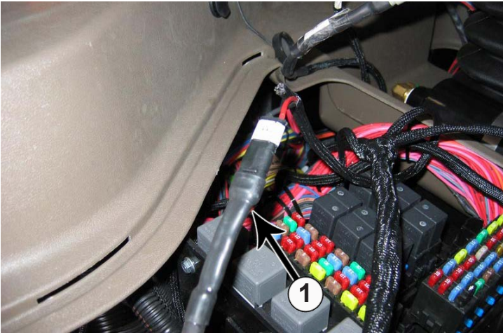
22. Connect the dozer angle extension cord (PN: 69-11663) to the wire harness (1). Run the cord through the hole in the floor of the fuse compartment.
